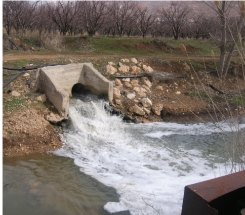
A DRAINAGE PIPE DISCHARGING IN THE RIVER, 1200 M FROM THE BARADA SPRING, ZABADANI AREA, FEBRUARY 2008
